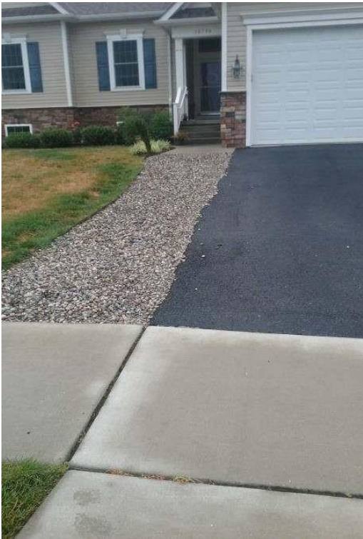
Driveway Border – Stones – does not comply with standard
