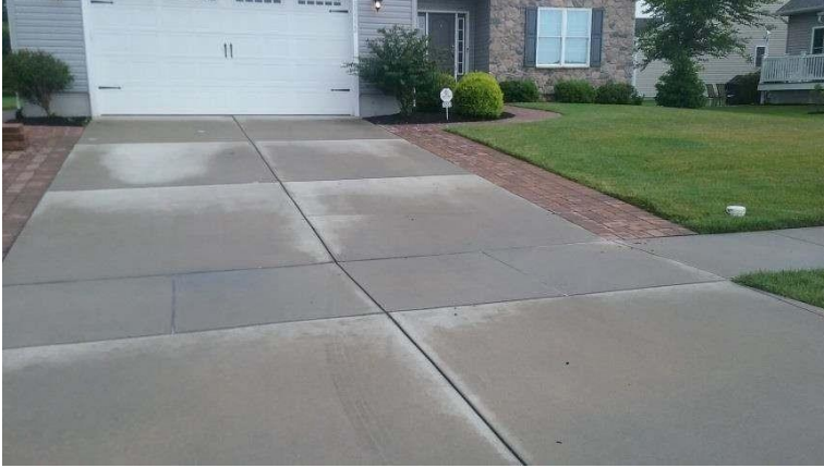
Driveway Border – brick – complies with standard
