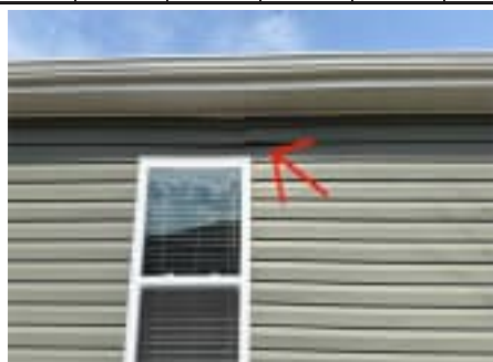
Loose Vinyl Siding
